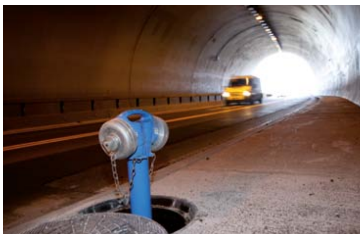
Raccordement incendie en tunnel
